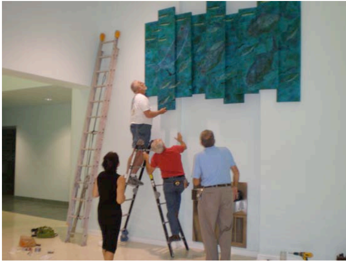
Artist Kim Workman and Director of Airports, Peter Horton supervise, as Ed Upmal and Bob D'Antonio install "Back Country" at the Key West International Airport terminal.
